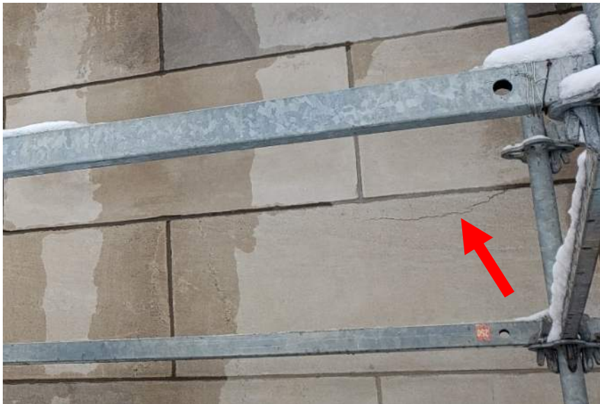
Figure 8. Enlarged image of Figure 7 showing a "half-moon" stone crack (red arrow).
