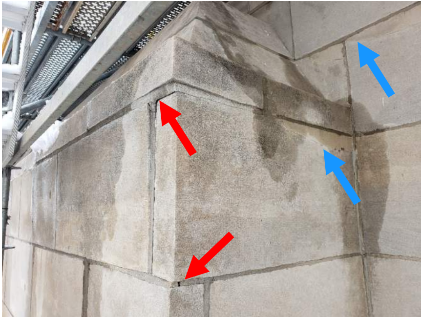
Figure 9. Locations of visible gaps at the stone mortar (red arrows) and “half-moon” patch repairs (blue arrows).
