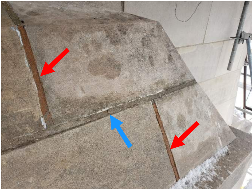
Figure 10. Locations of contrasting colored mortar (red arrows) and cracked mortar (blue arrow).
